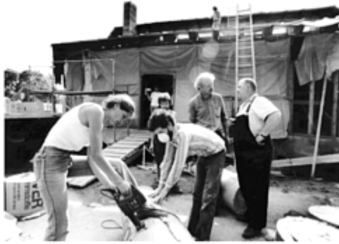
10.09 – Landau cultural centre: site work in progress, Peter Sulzer in discussion with self-builders.
