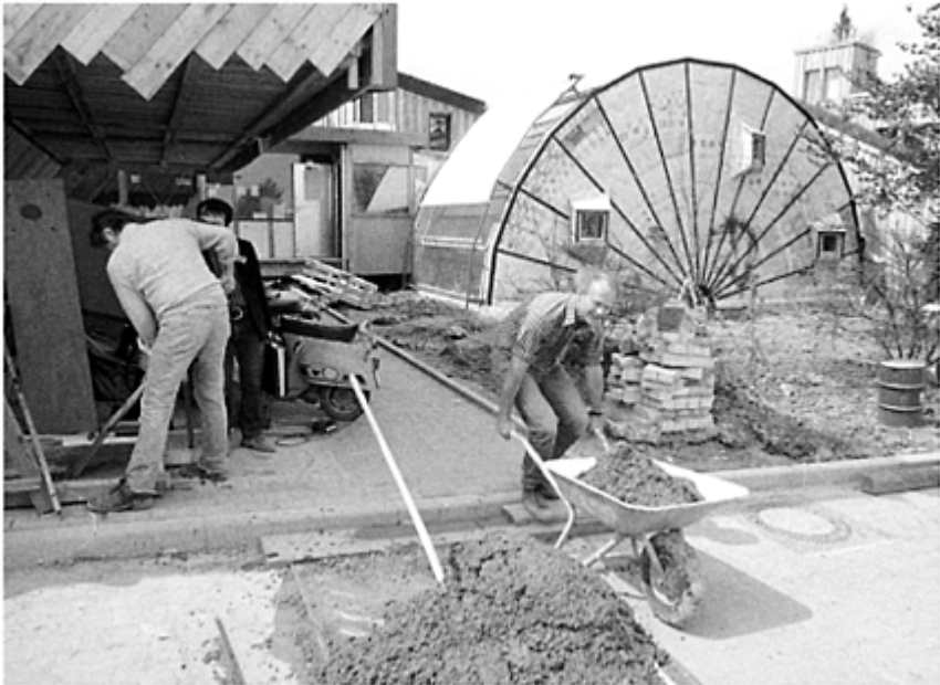
10.07 –Front of the Bauhäusle and path to the community building. Peter Sulzer is helping out with a wheelbarrow of concrete.
